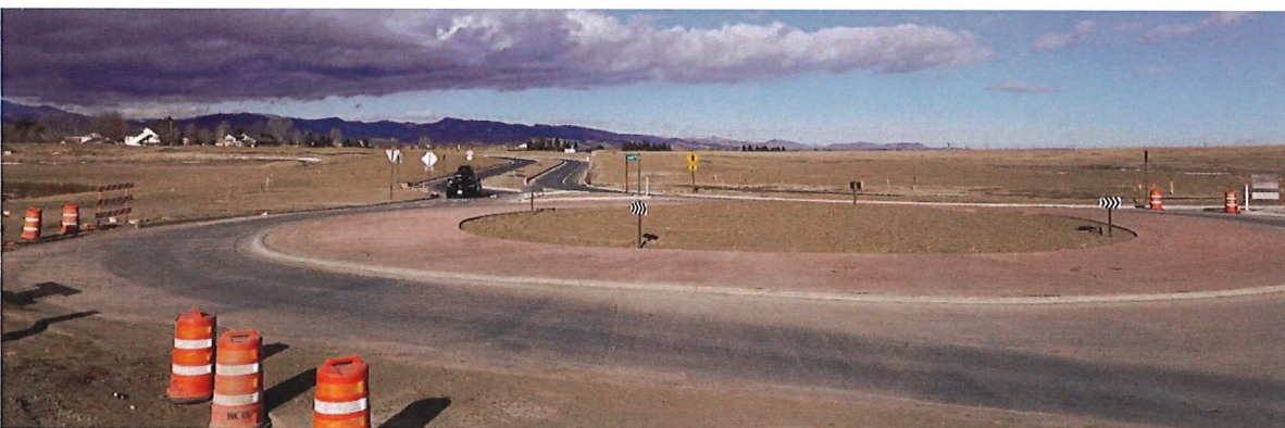
Top: New construction of Boyd Lake Ave Bridge over GLIC & new pedestrian box. Bottom: New alignment of Kendall Parkway.
